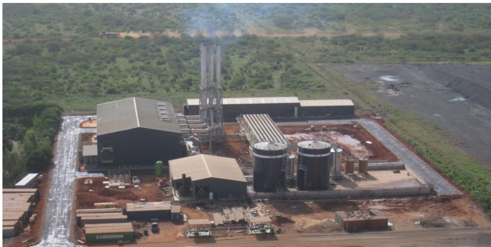
Les Ciments du Sahel S.A. cement plant pictured during the advanced construction phase of its MAN-fitted power plant. (source: Ingemas/TSK)
